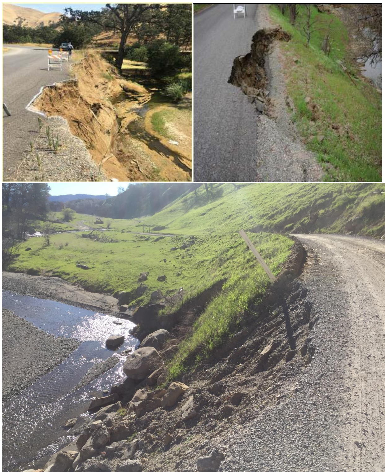
Figure 4-95 Streambank Erosion from 2017 Floods
