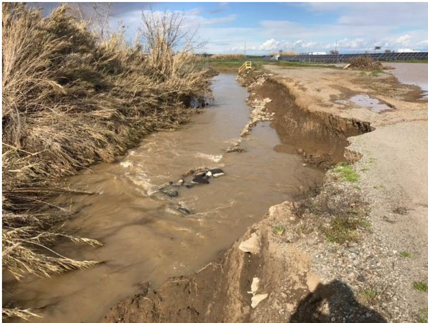
Figure B-16 City of Williams – Flooding near Wastewater Treatment Plant
