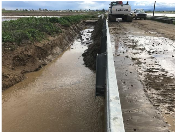
Figure B-20 City of Williams – Erosion Issues on Salt Creek
