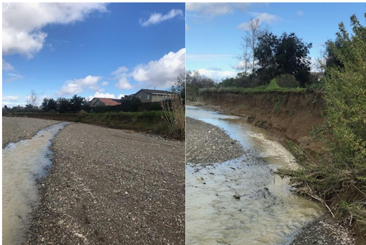
Figure D-9 CCSD – Streambank Erosion on Salt Creek
