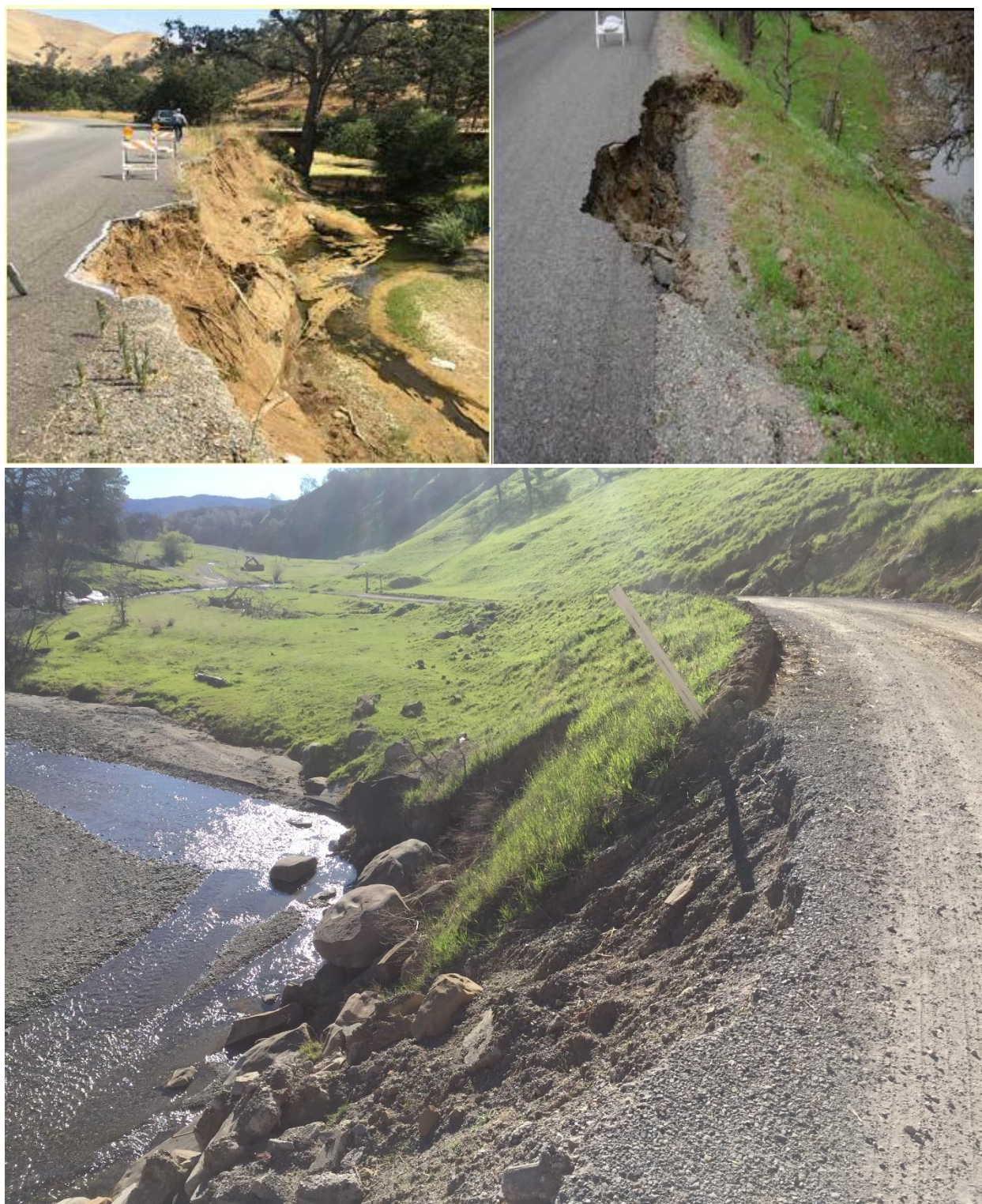
Figure 4-95 Streambank Erosion from 2017 Floods
